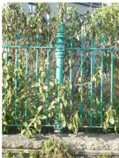
corroded newel post on southern boundary
