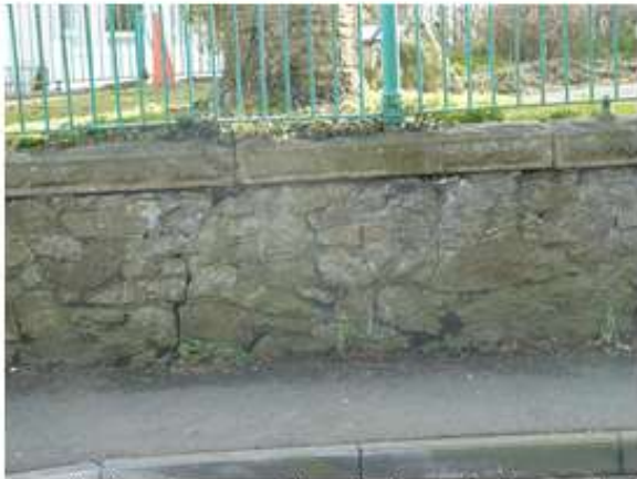
displaced masonry adjacent to Araucaria Araucana tree
