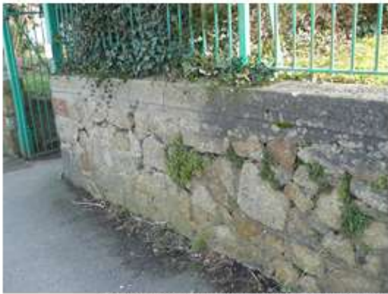
example of weed growth & defective pointing
