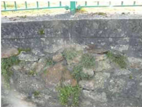
example of weed growth & defective pointing
