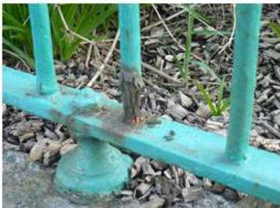
example of corrosion to metal railings
