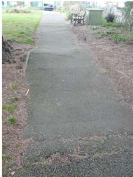
displaced tarmac adjacent to fir tree
