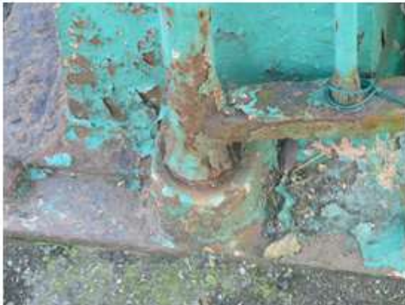
corrosion to east gate
